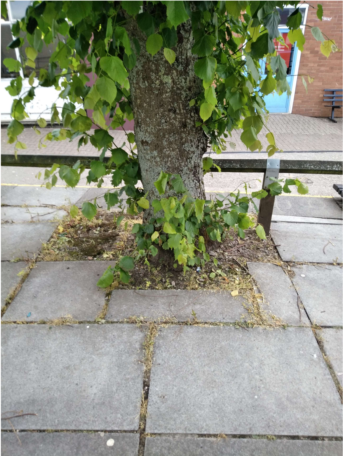
Photograph 9: T28 limited rooting area amongst hard surfacing, with evidence of root growth beneath the paving slabs.
