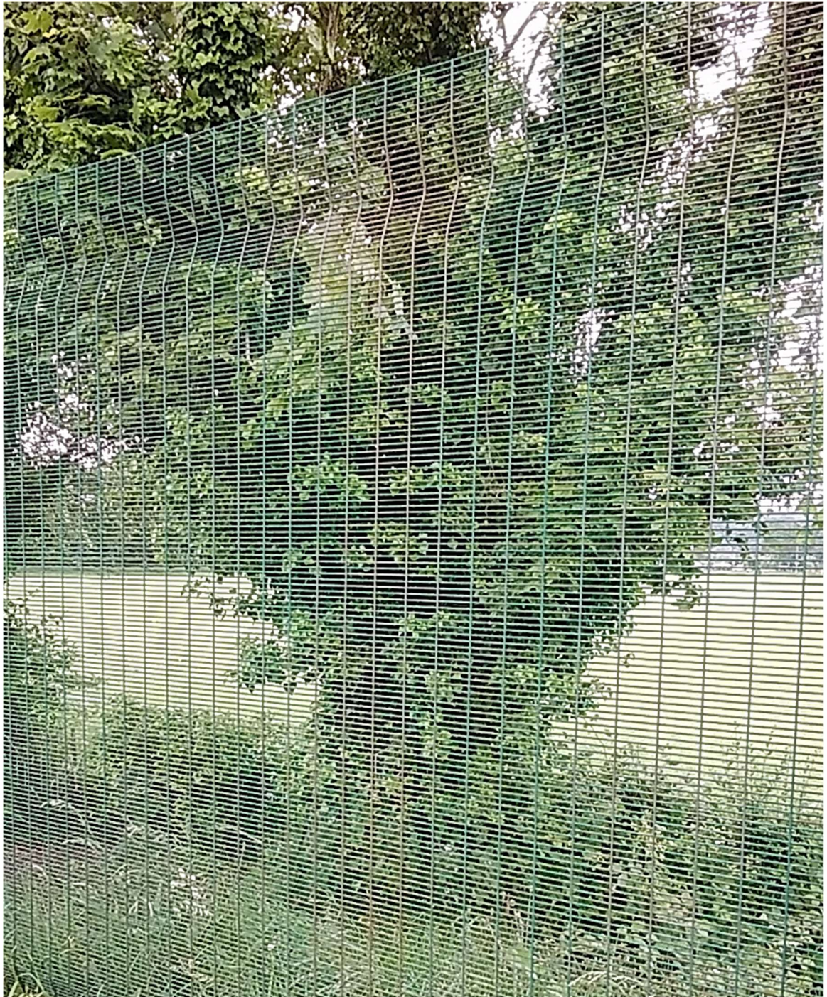
Photograph 4: T2 ivy clad stem restricts inspection of the base.
