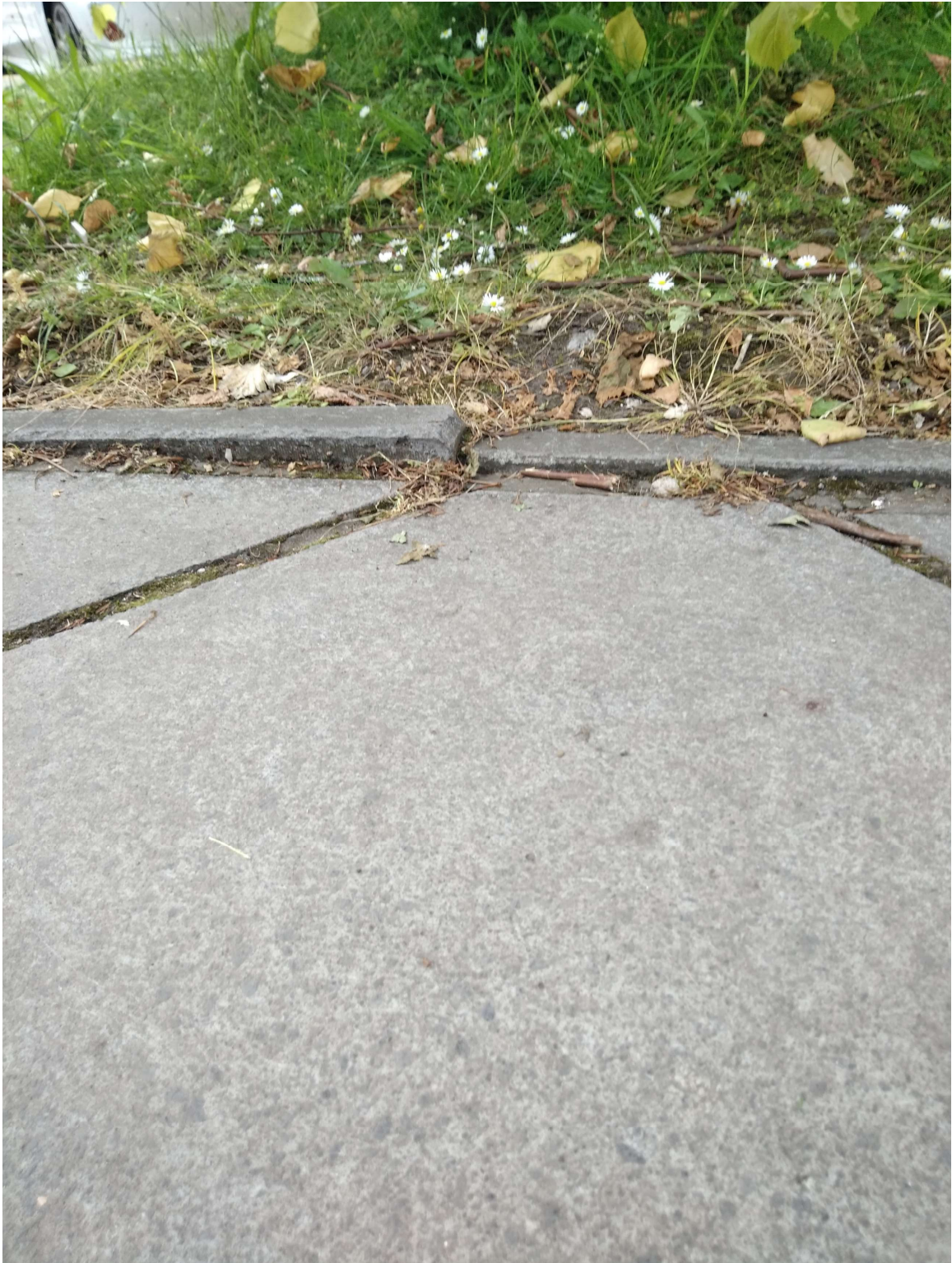
Photograph 7: T24 raised kerb stones due to root growth beneath the paved areas.
