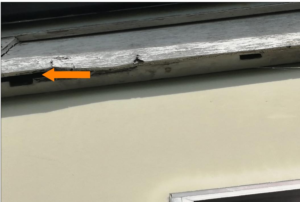
PLATE 21. Buildings D1 & D2 – Potential bat access points under fascia boards
