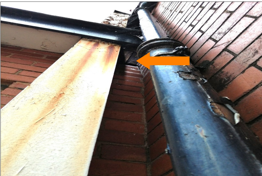
PLATE 9. Building A – Main sports Gym with bat PRF in corner of building join with Main ABC building (Target Note 6)
