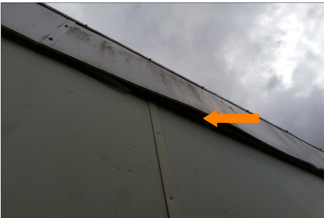
PLATE 19. Buildings D1 & D2 – Potential bat access points under fascia boards
