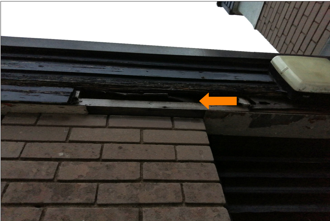
PLATE 11. Building H – Gym showing rotten soffit box (Target Note 8)
