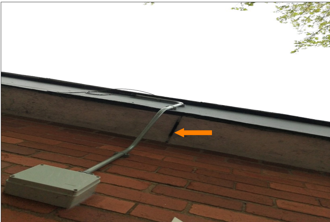
PLATE 5. Building K – Conference building rear showing gap in soffit box underside (Target Note 3)
