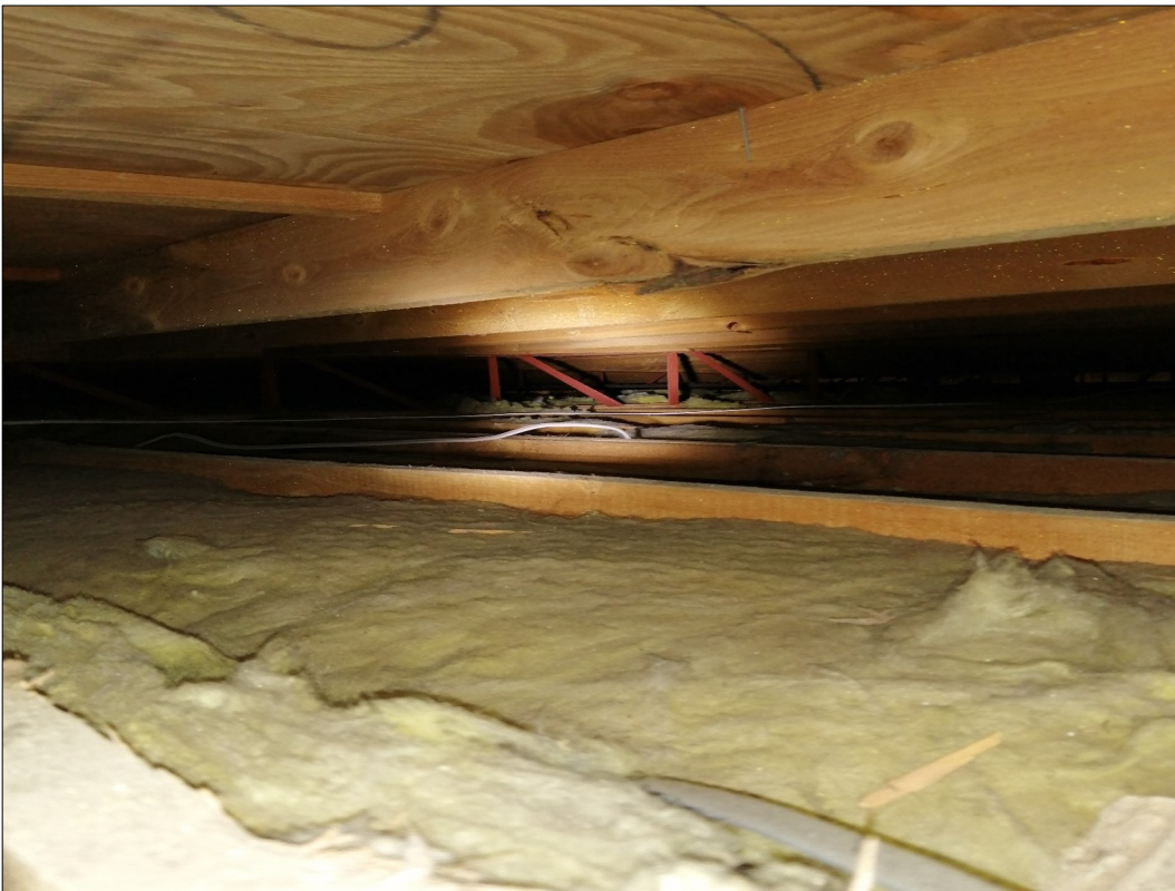
PLATE 24. Inaccessible narrow false ceiling roof voids in D1 & D2 buildings
