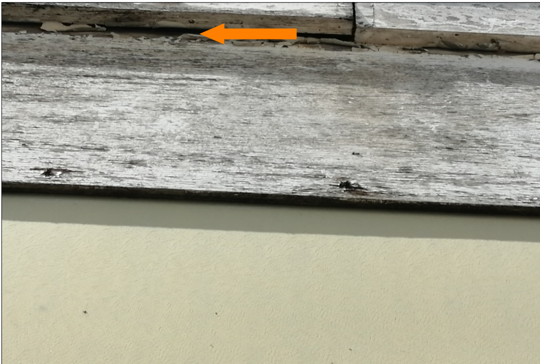
PLATE 20. Buildings D1 & D2 – Potential bat access points under fascia boards
